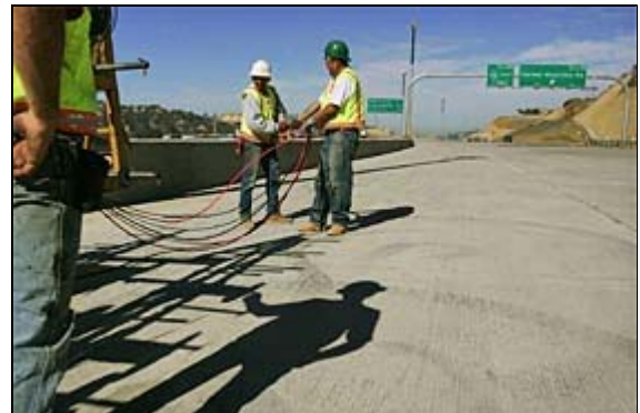
DAN TREVAN / Union-Tribune Working on wiring for lights near the new Carmel Mountain Road offramp from Interstate 5 last week were Sergio Delgadillo and Carlos Guzman. Construction will be completed soon on a bypass to state Route 56 to ease traffic for northbound drivers.
